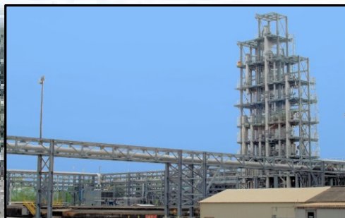
Pilot Solvent Test Unit
