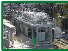
1 MW Membrane Pilot (MTR)
