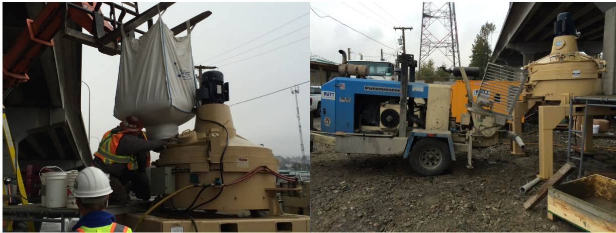
Figure 1: Concrete pan mixer and wet-mix shotcrete pump. After mixing, shotcrete was discharged into the shotcrete pump.
