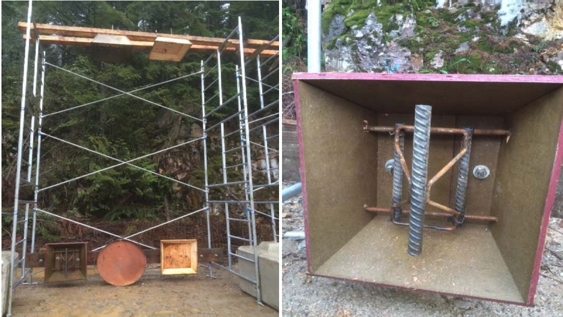
Fig. 4 Test panel set up for nozzleman qualification shooting for a section of lattice girder
