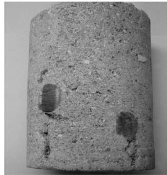
Dry-mix shotcrete, intersection #4 bars, linear defect from bar extending to back of panel. No interconnection detected or void against panel.
