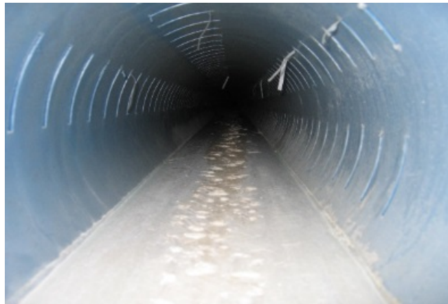
Figure 3: PP drainage pipe with precipitations. Picture: M. Testor, BEG
