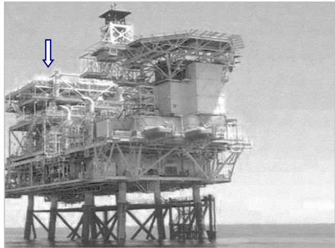
Fig. 9: Offshore platform with air coolers on top deck indicated by arrow.
