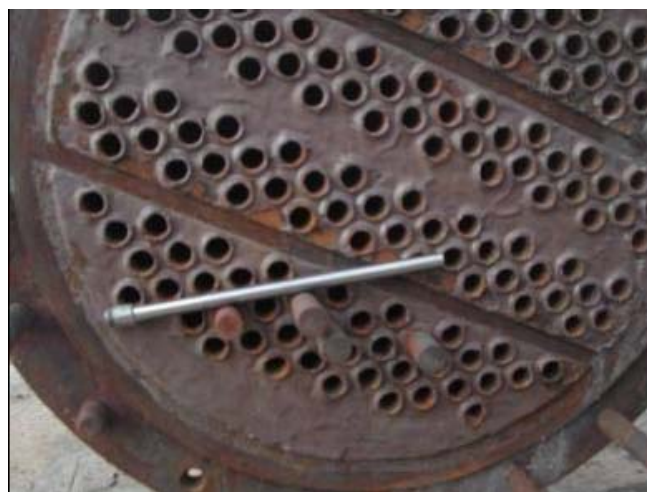
Fig.4: Clean H 2 S Cooler by CQM's ATCS
