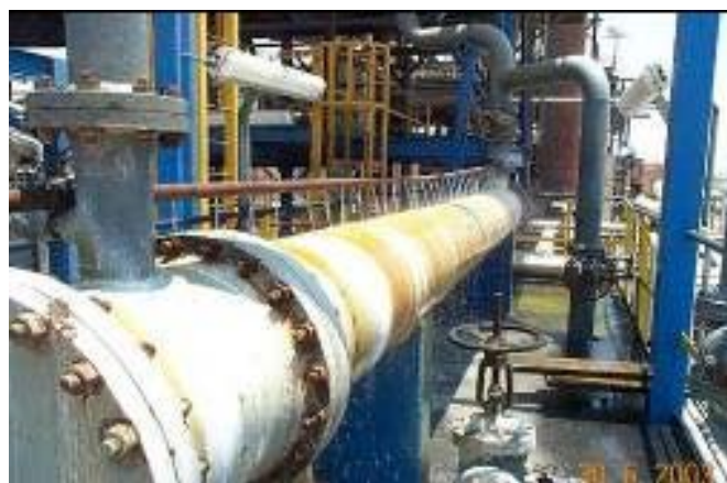
Fig.3: External cooling for the H 2 S Cooler
