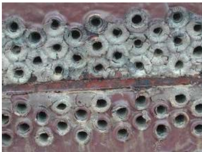
Fig 2: Clogged H 2 S Cooler: mud and scale
