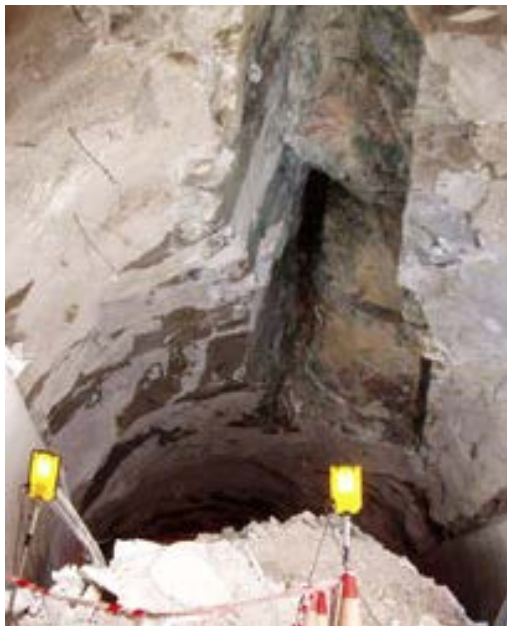
Figure 2 – Cave-in section of the fault zone
