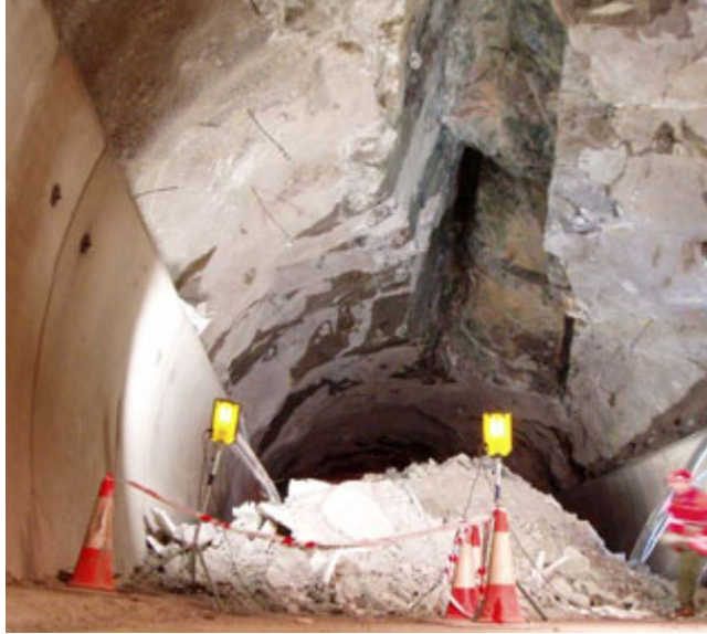
Figure 3 Cave-in section of the fault zone
