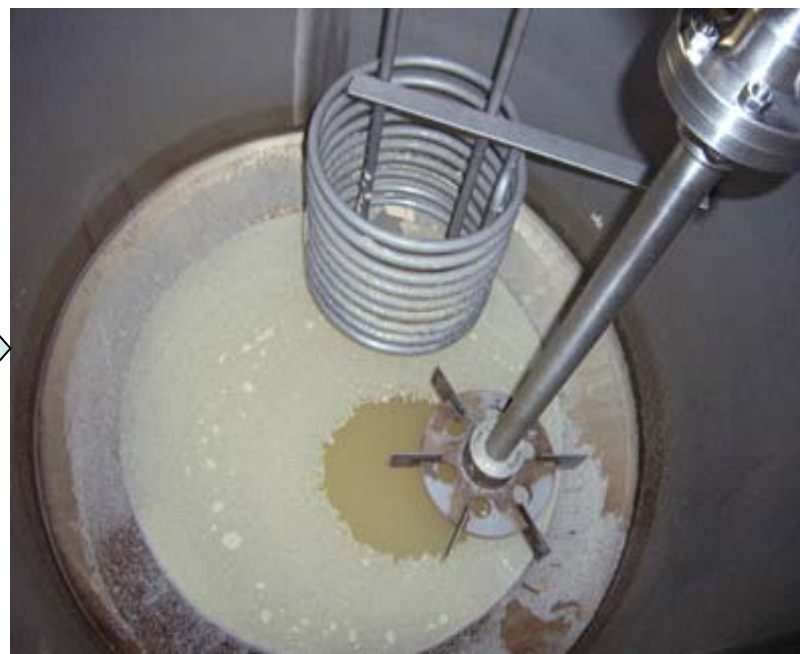
inside of mixing tank (right)
