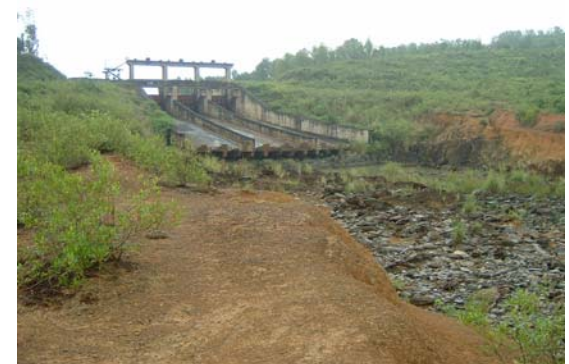
insufficient spillway capacity
