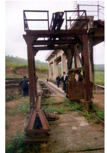
unreliable gate components
